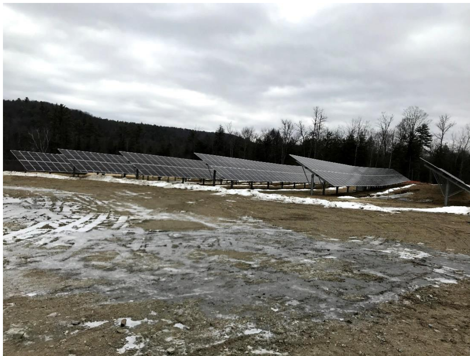
Grasse Rd Phase 1 Solar
