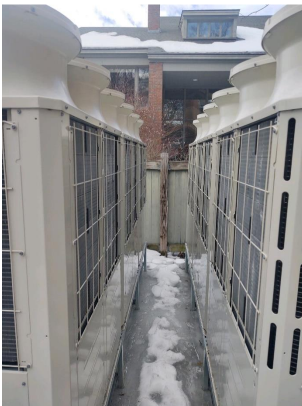
Howe Library Heat Pumps
