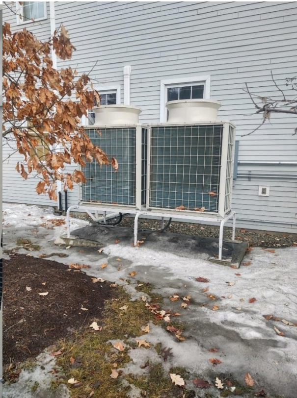
RW Black Heat Pumps
