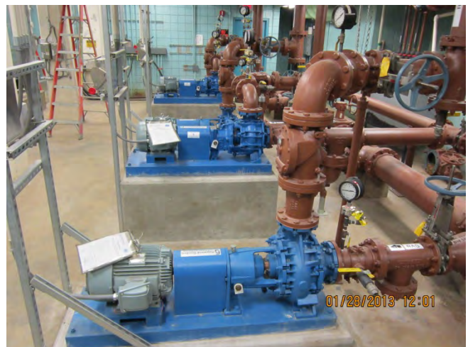
New RAS / WAS Sludge Pumps
