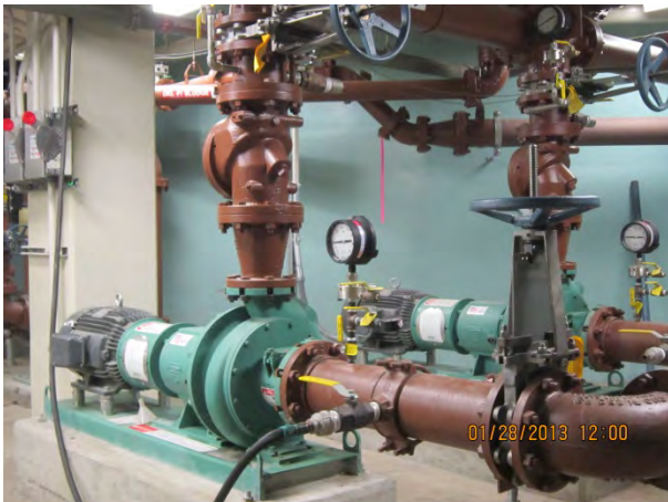
New Anaerobic Digester Mixing Pumps
