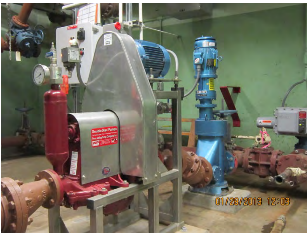
New Primary Sludge Pumps
