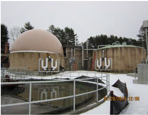
New Digester Covers and Methane Collection
