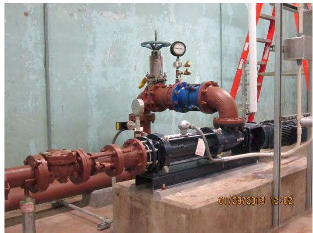
New Centrifuge Feed Pumps
