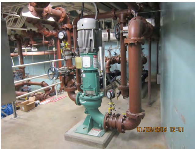
New Digester Recirculation and Transfer Pumps
