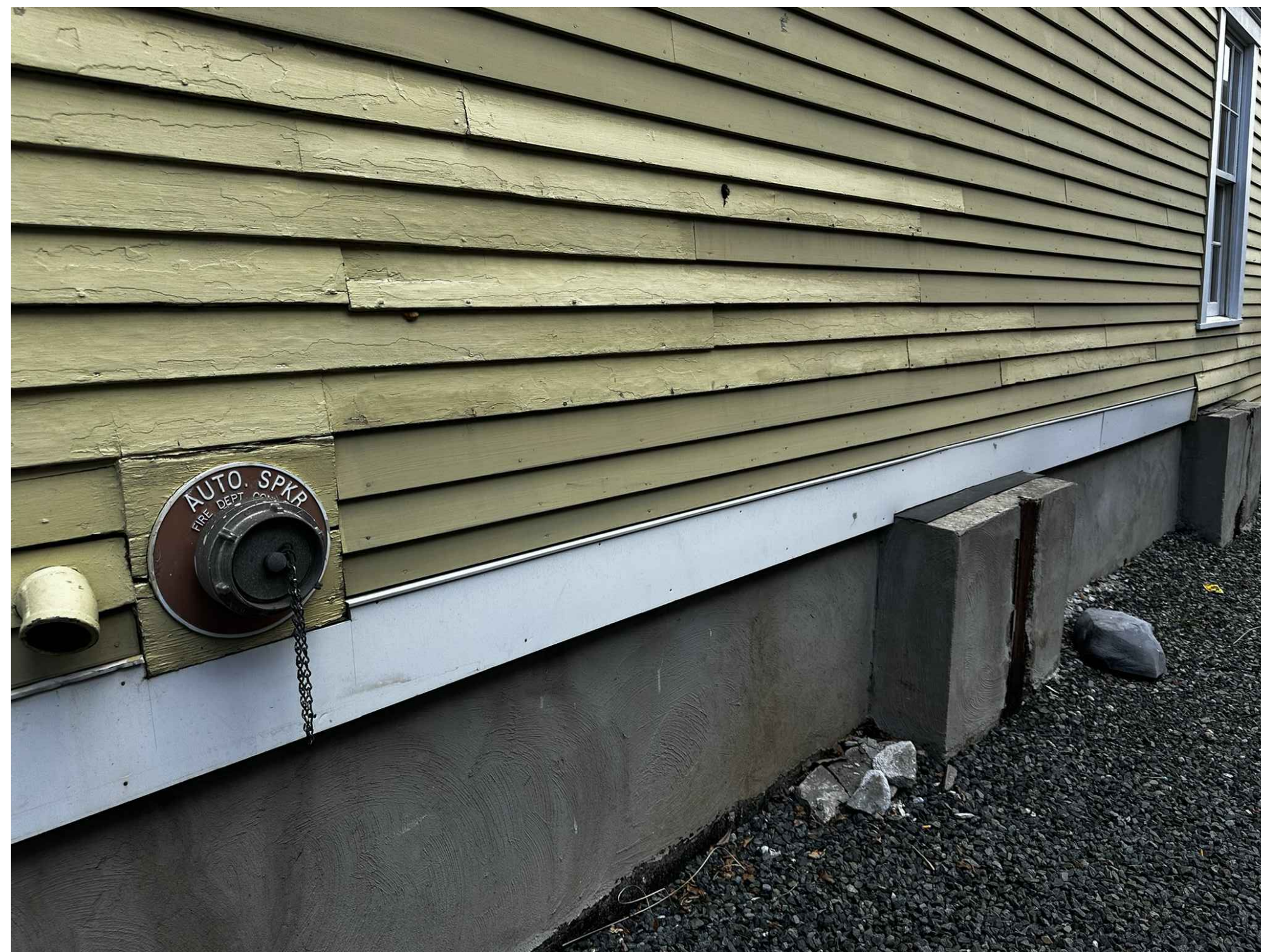
MAINTAIN CLEAR ACCESS TO EXISTING DRY HYDRANT ON LEDYARD BANK BUILDING, SEE SHEET L2.0
