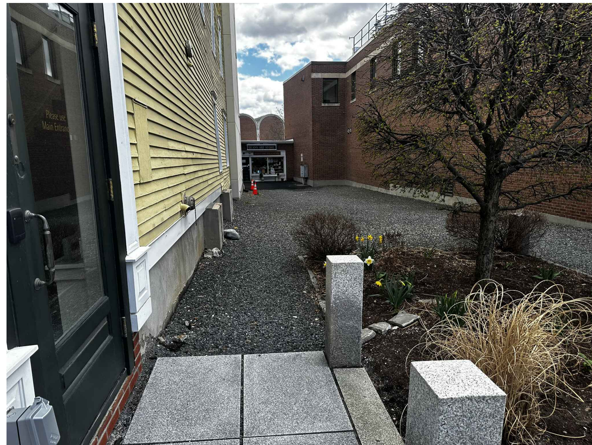
VIEW FROM LEDYARD BANK SIDE ENTRANCE MULCH BED AND ALL PLANTINGS TO BE REMOVED. ALL GRANITE POSTS, PAVERS, AND EDGING TO BE REMOVED, SEE SHEET L1.1
