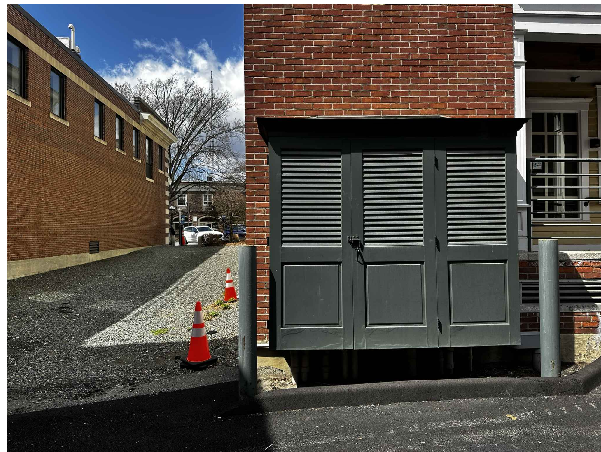
EXISTING ELECTRICAL ENCLOSURE FOR LEDYARD BANK AT BACK ENTRANCE OF PARK
